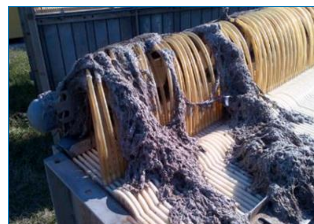
One of the types of fouling that hampers performance of the membranes at Gairloch WWTW
