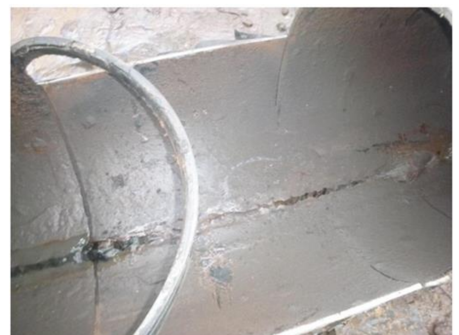
Showing Fracture along bottom of pipe
