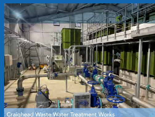
Craighead Waste Water Treatment Works
