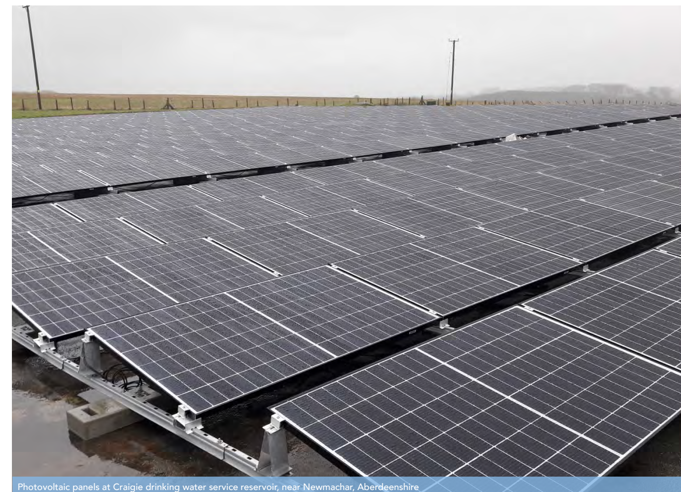
Photovoltaic panels at Craigie drinking water service reservoir, near Newmachar, Aberdeenshire
