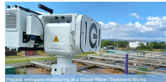
Process emissions monitoring at a Waste Water Treatment Works
